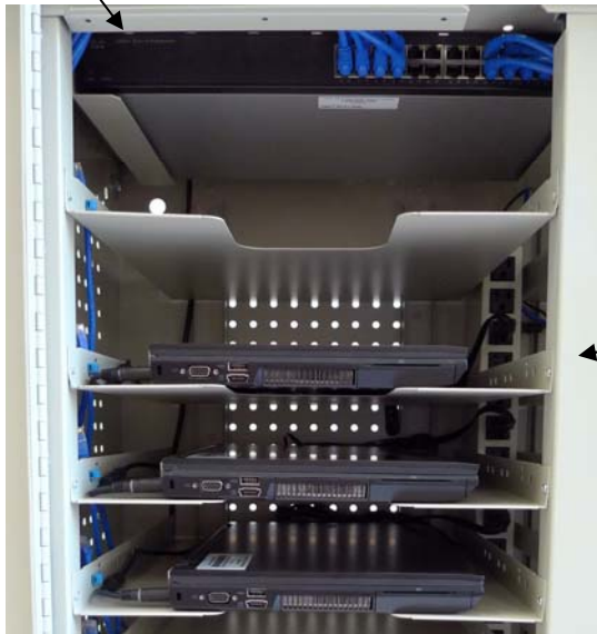
Ethernet cables all pre-installed neatly
