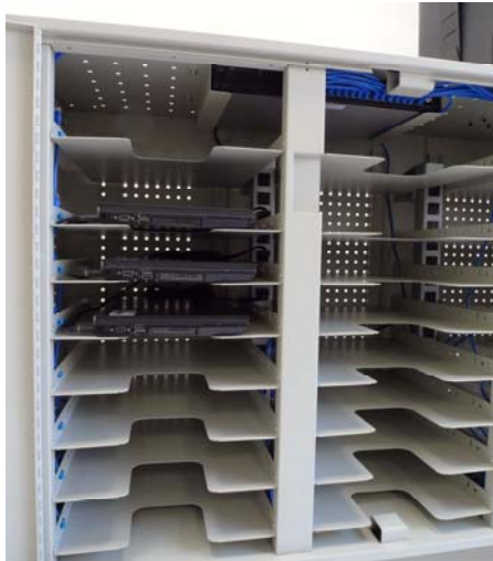
Ethernet cables all pre-installed neatly
