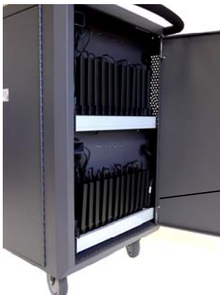
Power supply bricks and cabling in secure side compartment
